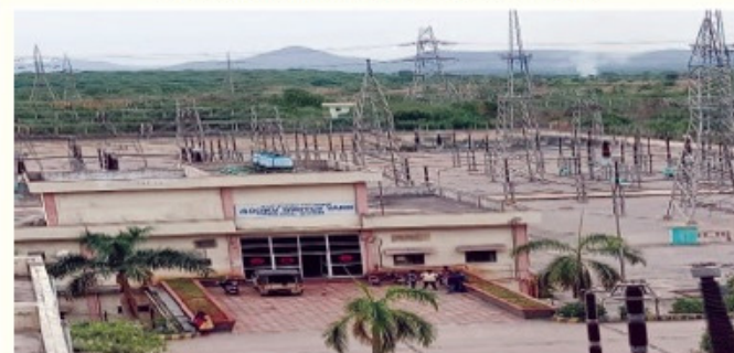
400 KV SWITCH YARD
